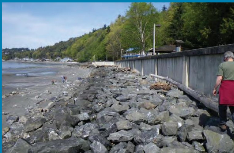
The current seawall and riprap at the north end of Seahurst Park; some parts will be removed in the next few years.
